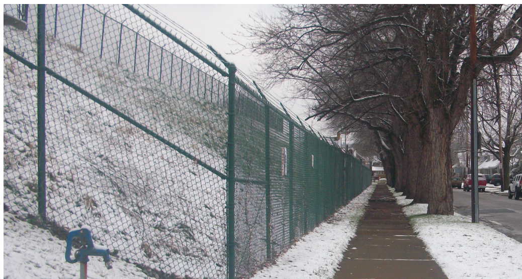
Outrigger installed incorrectly
